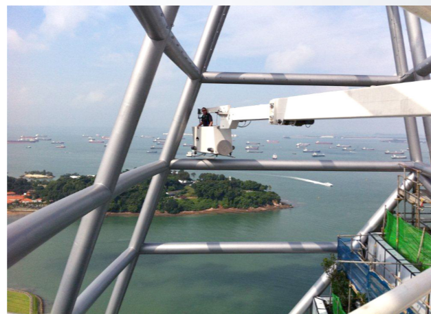
Top: The Shard, London (Top Machine) This page: Reflections, Singapore, multi-knuckle jib
